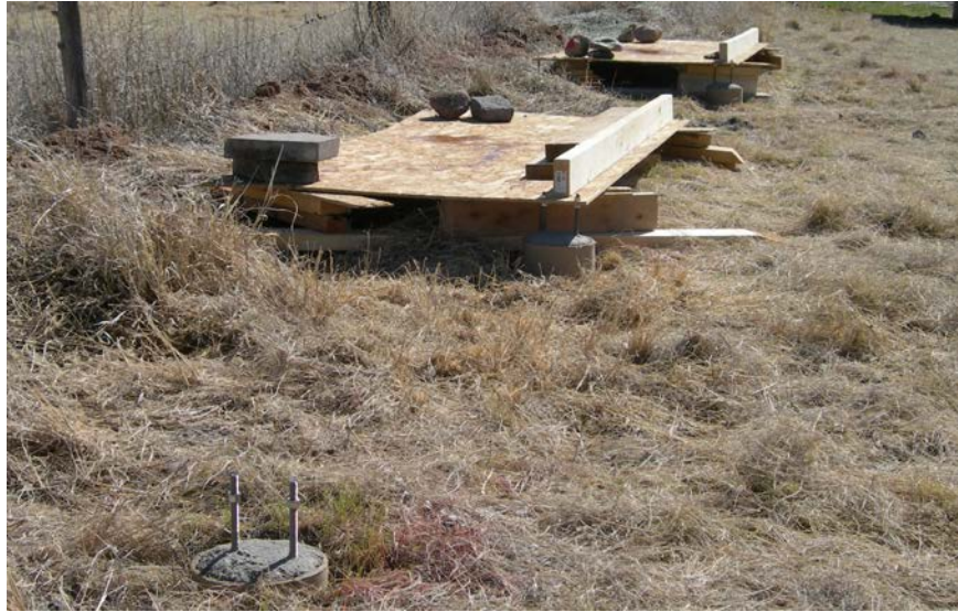
Figure 6. In the foreground, the two threaded rods for the right-front corner of collector number 2 are sticking out of concrete. The wood templates that temporarily hold the threaded rod in correct relative positions for collectors 3 and 4 are in the background.
