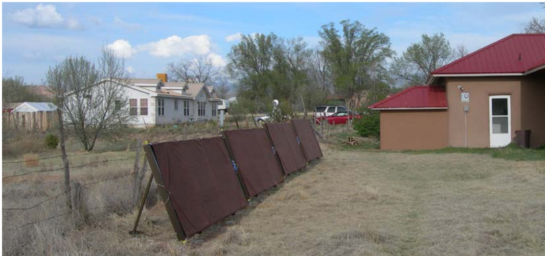
Figure 7. In the distance, the storage-tank shed is complete with sheet-metal roof and exterior plaster. In the foreground, the four collectors are mounted. From left to right: Collectors 1 and 2 are in series; collectors 3 and 4 are in series. These two sets are in parallel. (I covered them with canvas tarps during the year I was finishing the plumbing, even though the manufacturer said that was completely unnecessary.)
