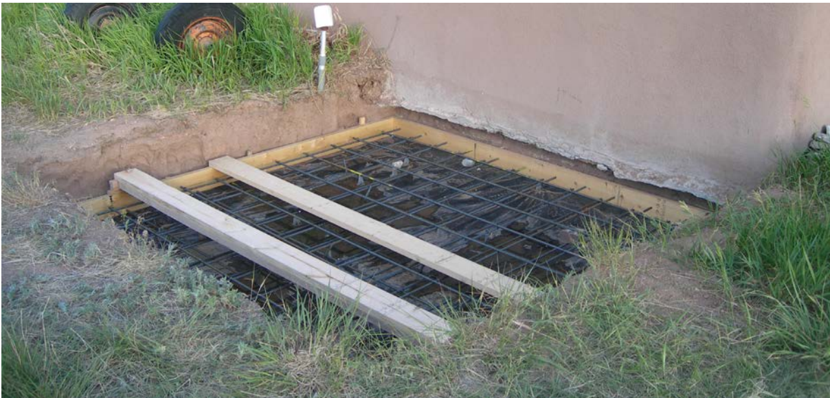
Figure 1. Rebar ready for pouring concrete to make the foundation under the storage tank.
