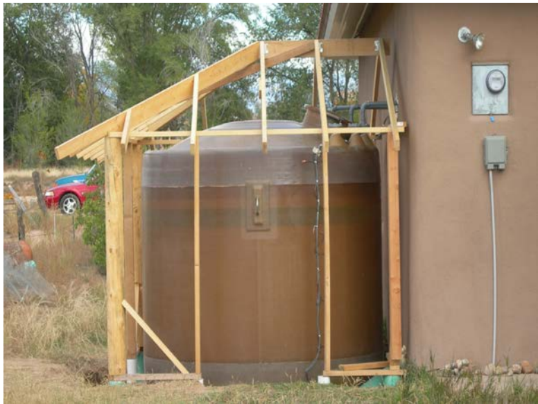
Figure 3. The tank in place atop the foam boards (which are out of sight below ground level), with pipes into the house and framing done.
