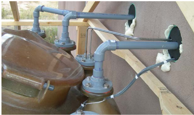
Figure 4. Details of pipe penetrations atop the storage tank. Thermistor wires also visible.
