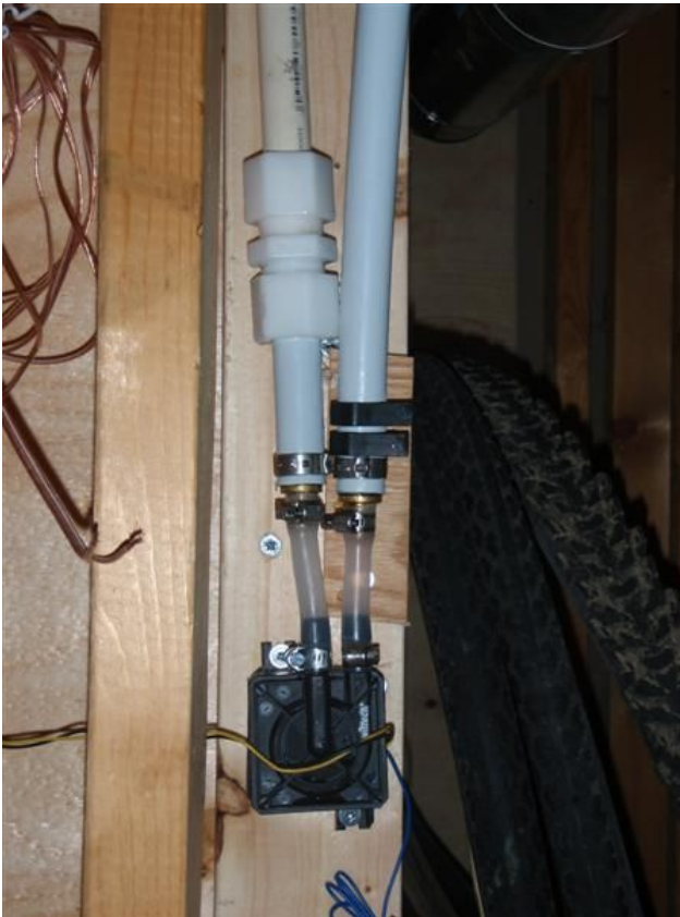
Pump (Swiftech MCP355) and 3/8" to 3/4" piping arrangement
