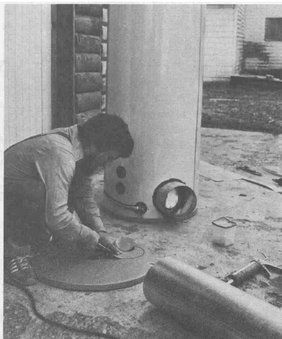
Photo 10-2: Round boots are attached to the top end cap and to the jacket low on the tank. The boots are placed to be more or less opposite each other, and all holes in the jacket are covered with sheet-metal scraps and sealed with silicone. This exchanger was built using a water-filled coil of \frac{3}{8} -inch copper pipe spiraling around the tank inside the jacket. In our tests it didn't perform as well as the fin type.
