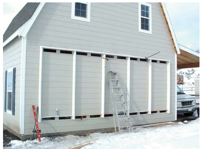
The frame is mounted on the outside wall after the vents are cut.
