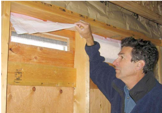
The author inspects the thin plastic flapper valve that prevents reverse airflow and helps keep heat inside the building.
