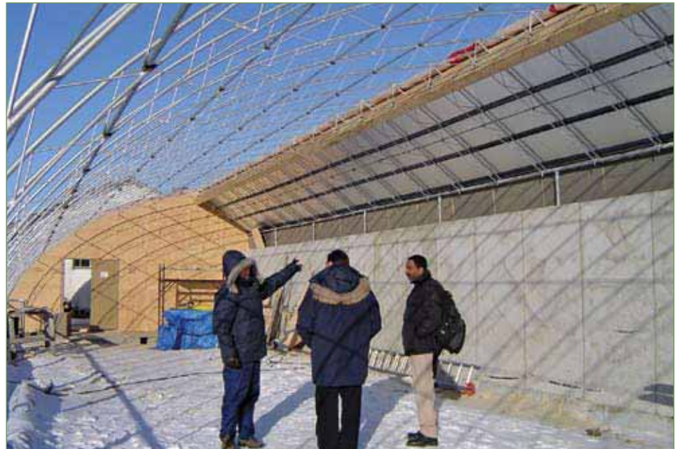
Solar greenhouse under construction at St. Francis Xavier, Manitoba. The rear wall is concrete, a variation of the sand-filled wall used in the greenhouse at Elie.
