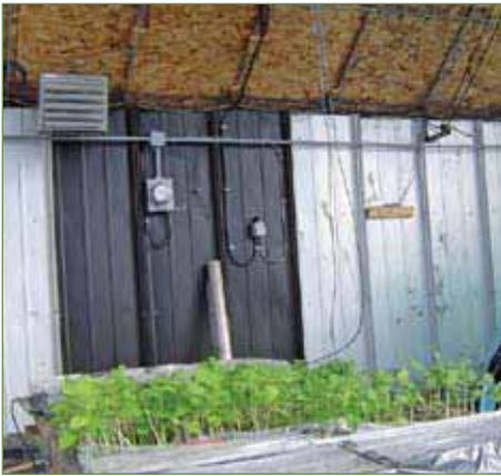
Second chamber in the greenhouse at Elie, February 7, 2006. One of two 5-kW GX agricultural electric unit heaters, top left, helped keep plants warm. Note section of rear wall, painted flat black to absorb solar heat.
